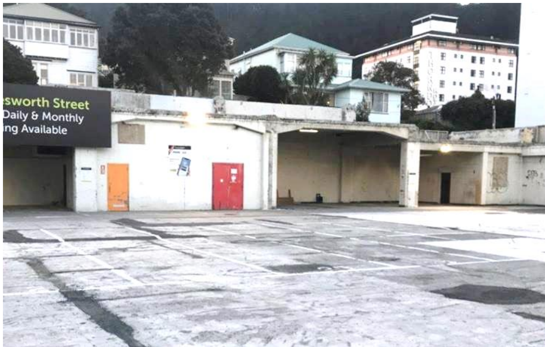
Photograph 3: View of northwest corner of the site showing, left to right, the enclosed substation, the former plant room which was originally enclosed and, through the door, the fuel oil tank room.
