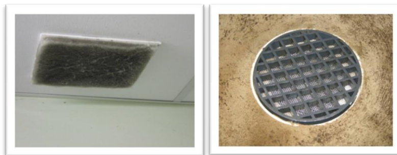
Photos 4 and 5: Airflow and water flow exit points are all covered with fine mesh.
